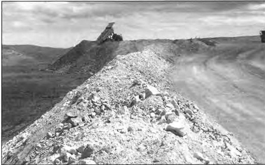
Figure 11.3-4 A truck is dumping an upper lift onto a lift that is actively under leach. The road formed by haul truck traffic on the heap can be seen on the right.
